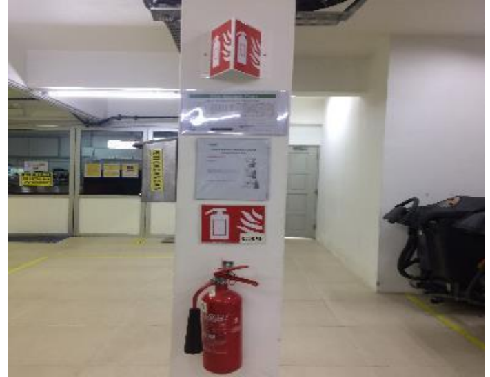
Evacuation escape map, fire extinguisher and usage guidelines clearly displayed and accessible.
