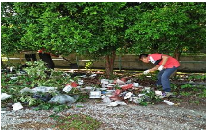
Fallen leaves, branches and rubbish were removed from the drain to allow rainwater to flow freely and not stagnate the drain.
